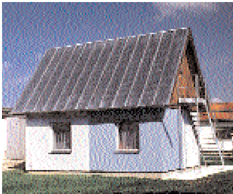
The research scientists tested the function of the moisture barrier on a building with a sheet metal roof.
